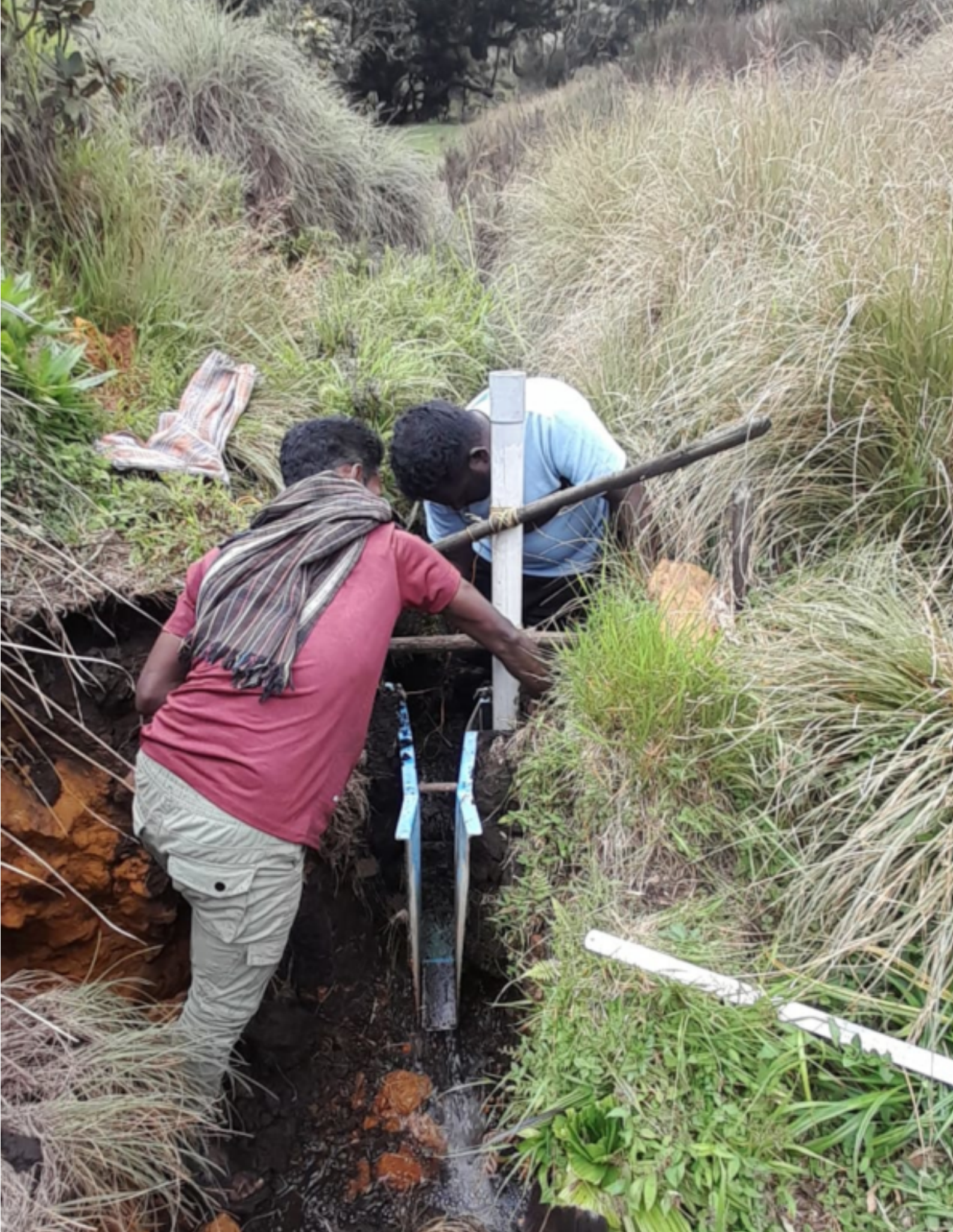
Flumes were installed to measure stream-flows during the dry periods.
